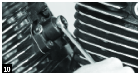
10 Next, he preassembled the cam chain tensioner per the Kawasaki Service Manual, and installed it in the front cylinder.
